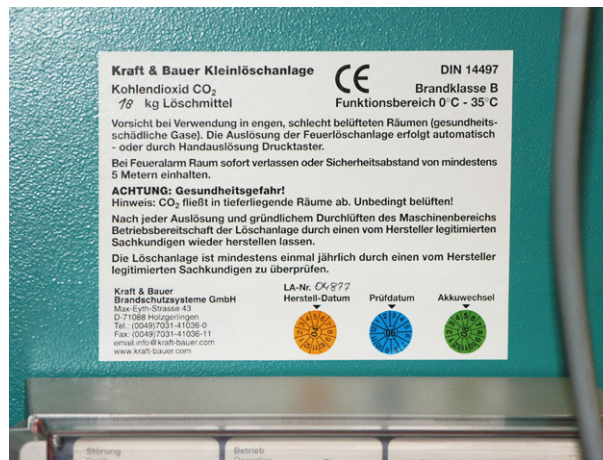
Example: Inspection stickers Kraft & Bauer
